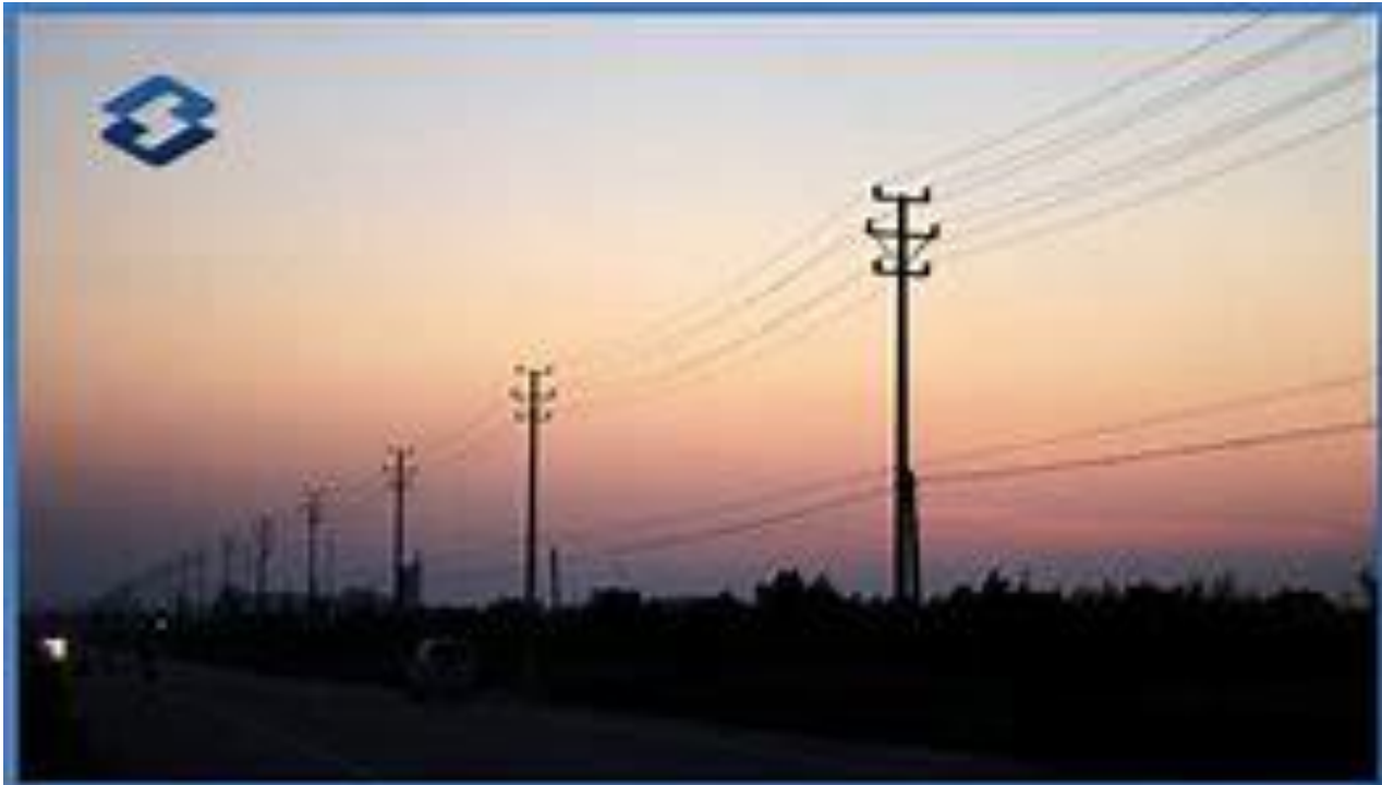
132 KV (29m high)
