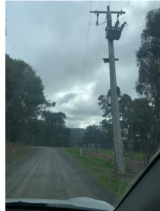
22 KV Distribution line
