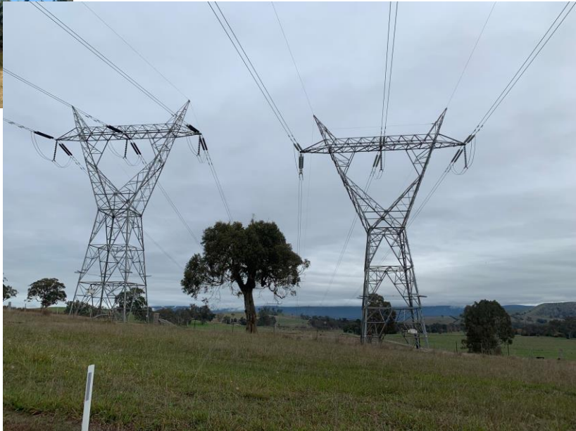
Duel 330KV National Grid near Molesworth (35-40m high)
